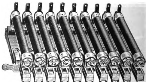
FIG. 220.—Strip of Cook heat coils arranged for use on a cable terminal.
